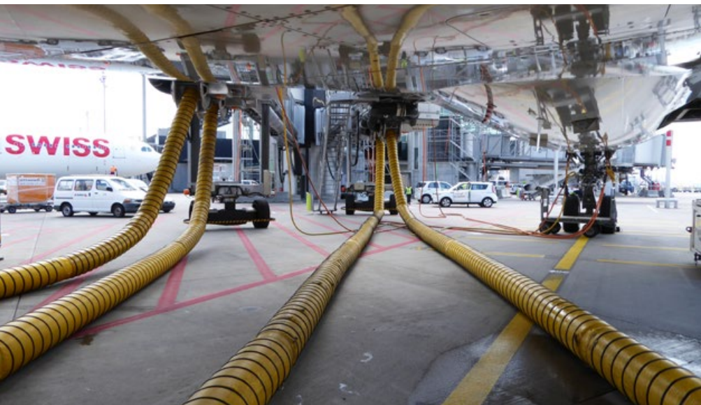
The yellow hoses supply conditioned air from the pier into the aircraft, which is also provided with stationary electrical energy.
