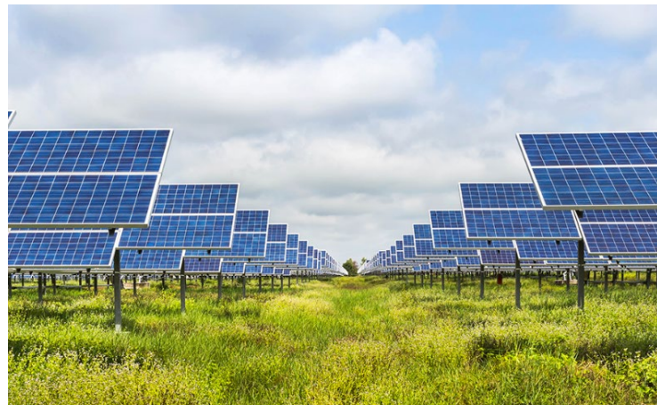
Solar power Plant
